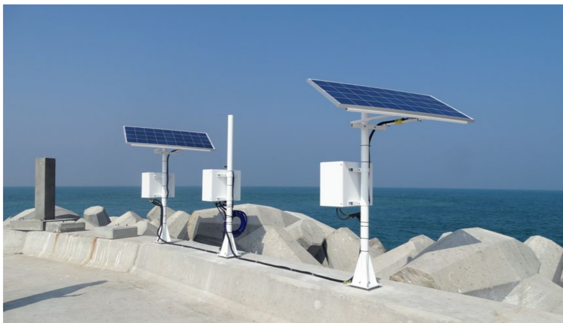
Automatic Marine Stations System for a client in Oman, specifically focusing on Wave and Current Stations, with the onshore installation including the jetty portion at the shore of the Arabian Sea.
